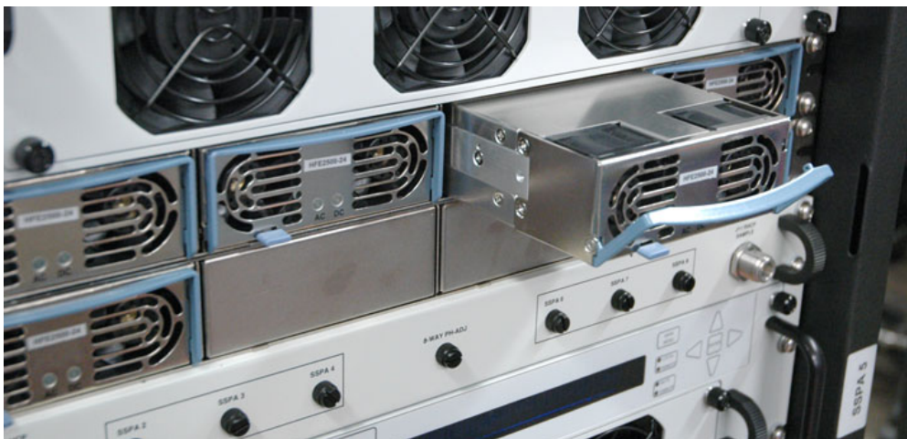
Figure 6: N+1 Power Supply
