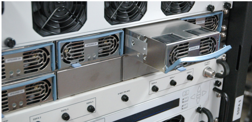
Figure 24: N+1 Power Supply
